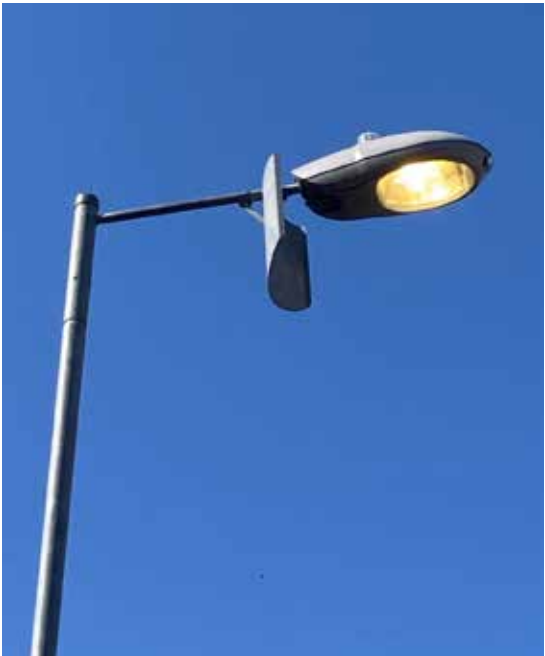
Well-performing WRTL Arc/Cosmo columns
